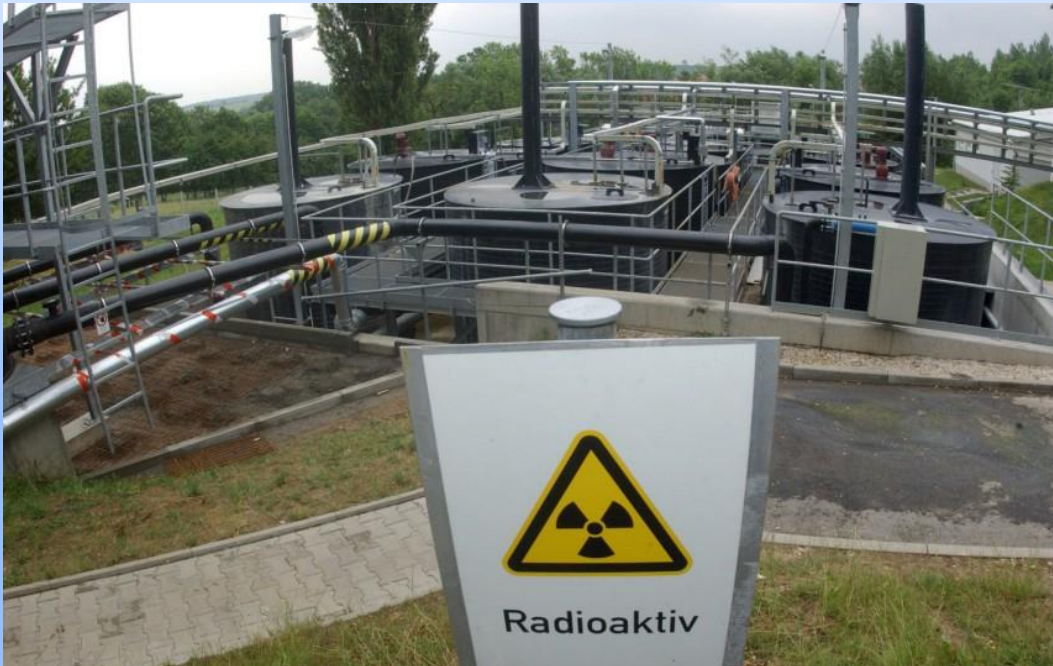
Water treatment plant Seelingstädt (Thuringia) of the federally owned WISMUT Limited liability company (GmbH) (photo: picture alliance / dpa)
